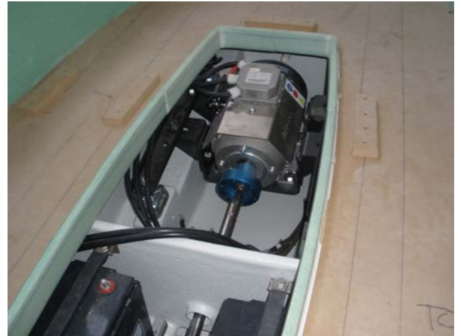
Motor and battery installation
